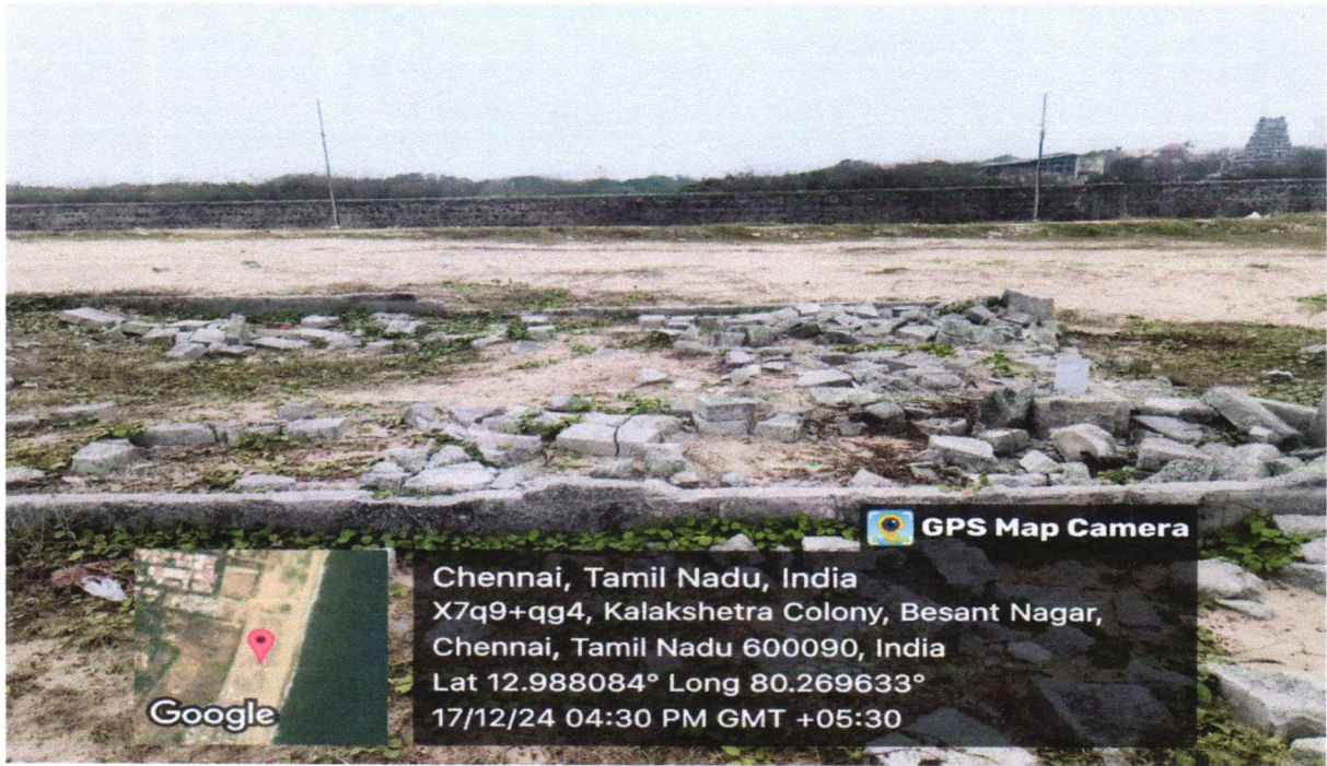
Fig 7. Dilapidated Construction near to the Arupadai Veedu Murugan Temple in Besant Nagar's Kalakshetra Colony in Chennai (Tamil Nadu)
