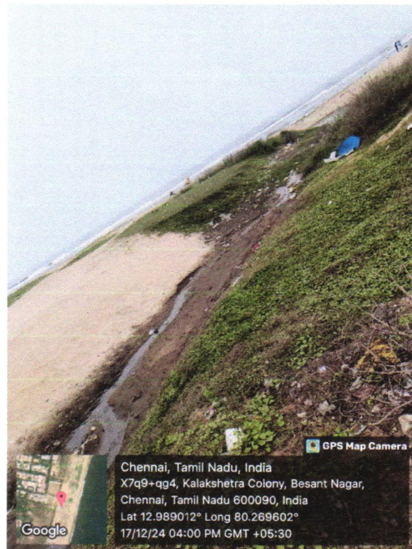
Fig 9. Natural Drian for rain water was observed near to the Arupadai Veedu Murugan Temple in Besant Nagar's Kalakshetra Colony in Chennai (Tamil Nadu)
